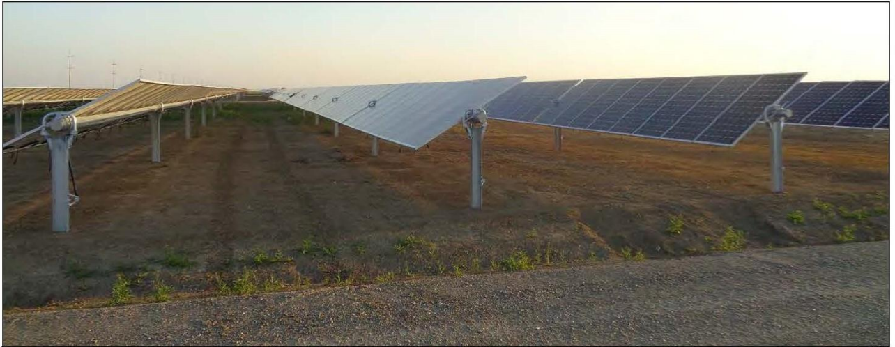
Solar PV Modules on Horizontal Trackers
