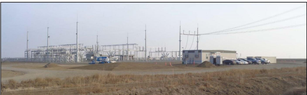
Photo 6: Typical 230-kV Project Substation with O&M Building
