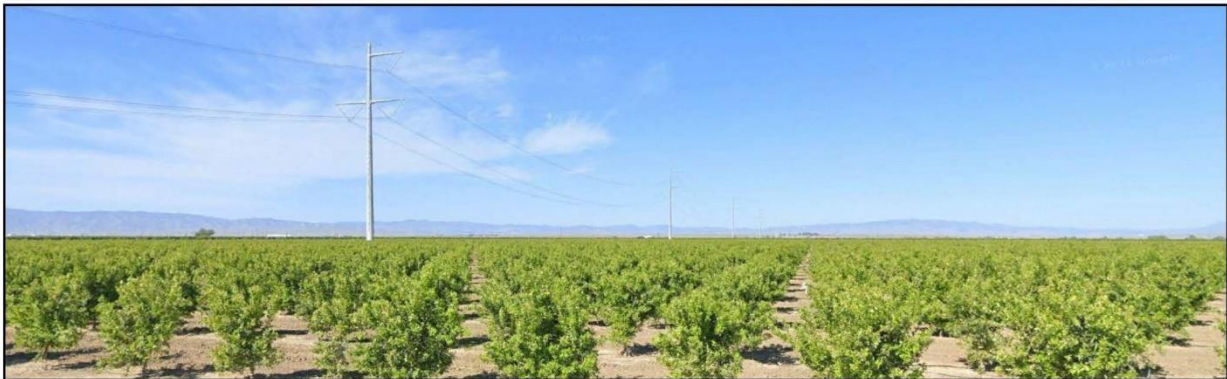
Photo 5: 500-kV Transmission Monopole Line
