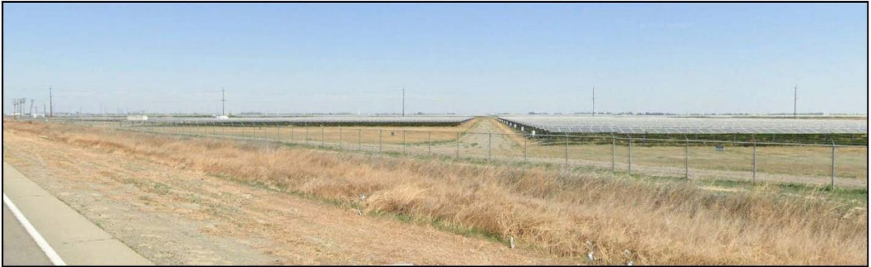
Photo 1: Typical Solar PV Field
